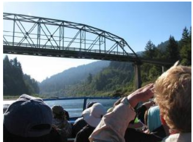
The river flowed over the deck of this bridge in the year of the highest recorded flow.
